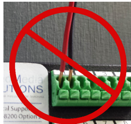
DO NOT DO THIS! No bare wire should extend beyond face of port.
