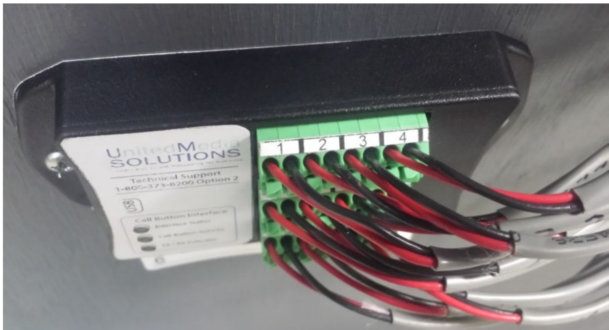
Top view of mounted interface. Note that no bare copper is exposed.
